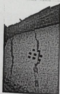
Figure 3: Cracks in the walls of the house due to the blasts in the mines.
